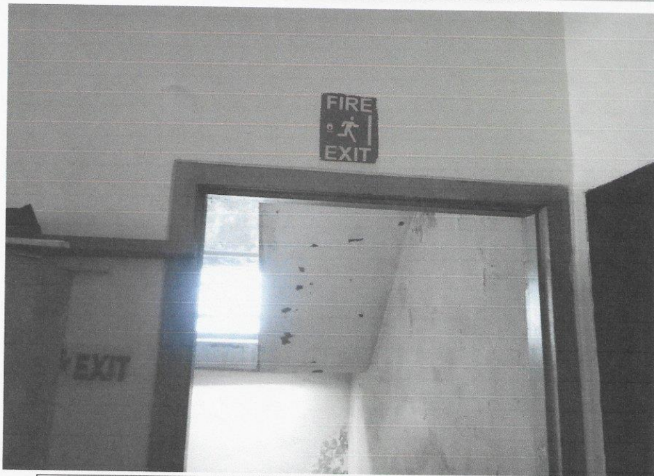
EMERGENCY EXIT SIGNAGE AT COLLEGE OF ENGINEERING AND ARCHITECTURE BUILDING
