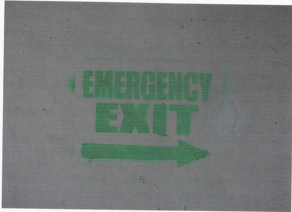
EMERGENCY EXIT SIGNAGE AT MAIN BUILDING
